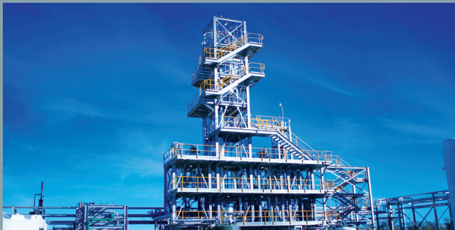
HCl, HBr AND H 2 SO 4 SKID-MOUNTED UNITS
