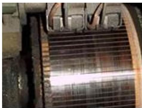
Figure 1 - Effects of grease (from bearings) on a commutator machine
